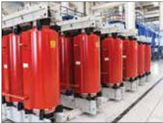
Dry Type Transformer
